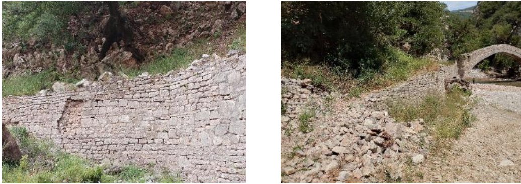
Image 3-59. Damage to the stone-built retaining wall of the path leading up to the bridge from the east. Source: NTUA Research Team, 2023.
