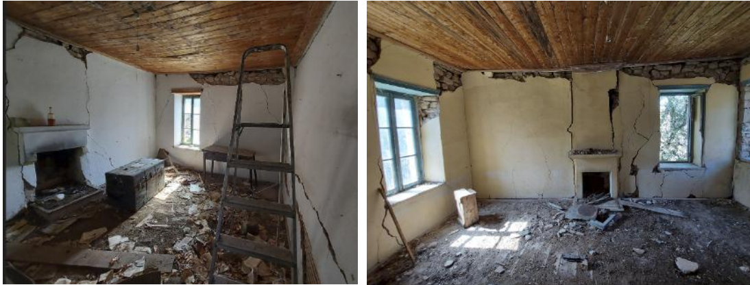
Image 3-55. House "of the Teacher". Cracks due to out-of-plane bending of the transverse walls. Source: NTUA Research Team, 2023.
