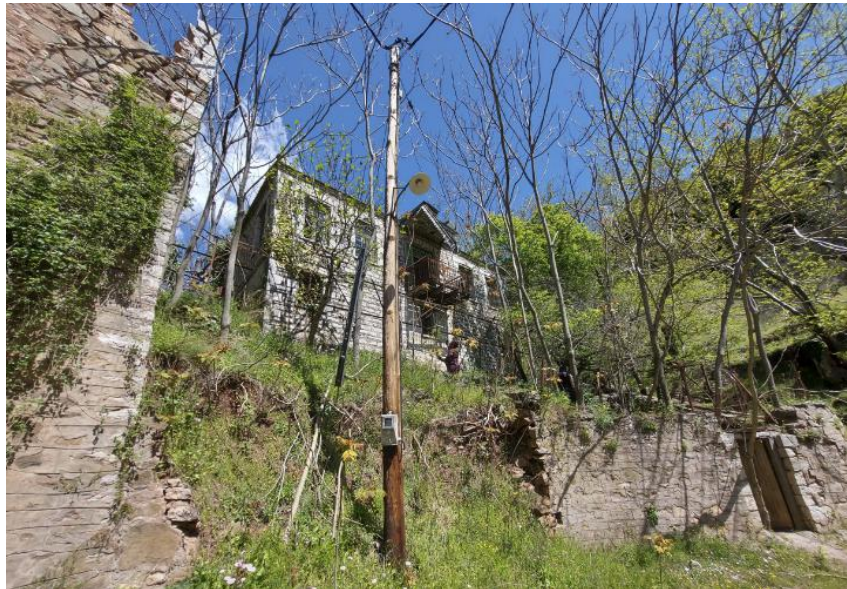
Image 3-28. Karageorgos House. The retaining wall at the property boundary is visible, part of which has collapsed. Source: NTUA Research Team, 2023. Drawings: A. Vienna, A. Zacharaki, Z. Kondyli, N. Sakka, V. Laspia, O. Spyridaki, A. Stefani, D. Christou, postgraduate students of the MSc "Monument Protection" NTUA.
