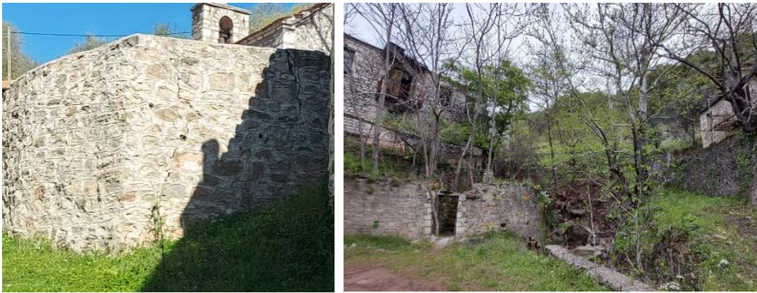
Image 3-47. Retaining walls with significant damage. Source: NTUA Research Team, 2023.
