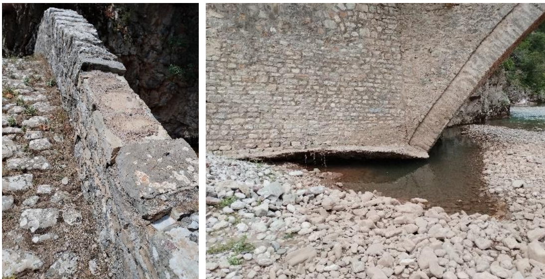
Image 3-57. Loss of stones in the parapet of the bridge. Source: NTUA Research Team, 2023.
